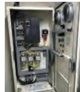
Renewal of the plant air-conditioning units to inverter control (control panel) system
