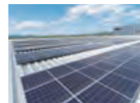
The solar power modules installed on TATSUTA Technical Center's plant building
